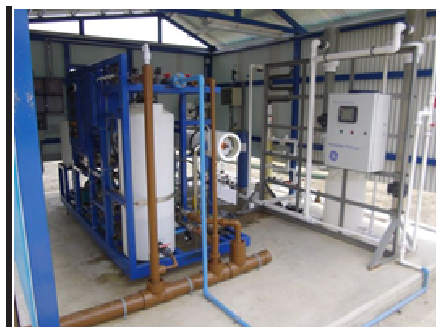
b: SWRO pilot beach well monitoring
