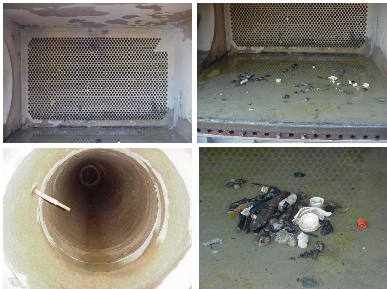
Figure 4.14: Pictures of the as found condition of the condenser during the biocide trial
