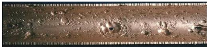
b: practical occurrence of steel corrosion causing red water and perforation
