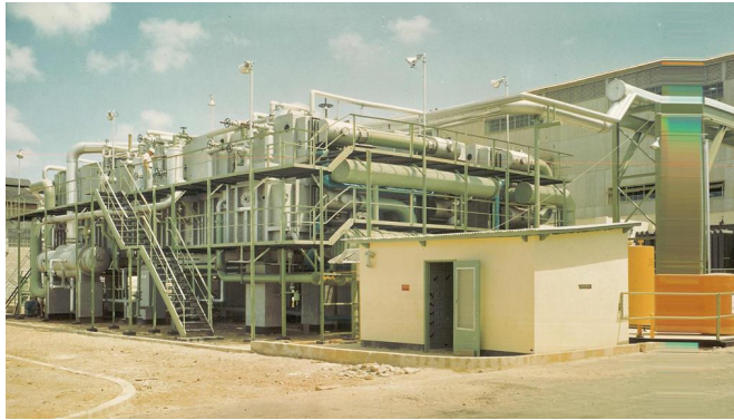
Figure 2.27: The first MSF desalination unit at W.E.B. Aruba N.V. in 1965 [2.5]
