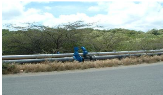
Figure 7.30: An up-ground water transport-line with flushing facility at the South coast of Aruba
