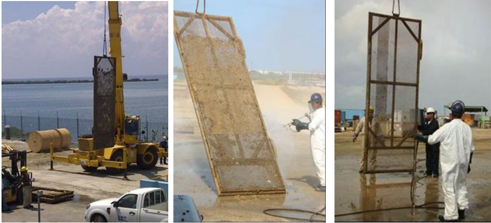
Biofouled intake screen Hydro blasting intake screen Cleaned intake screen Figure 4.4: An intake stationary screen before, during and after hydro blast cleaning
