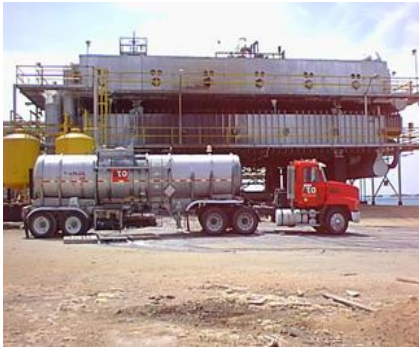
a: vessels' surface corrosion
