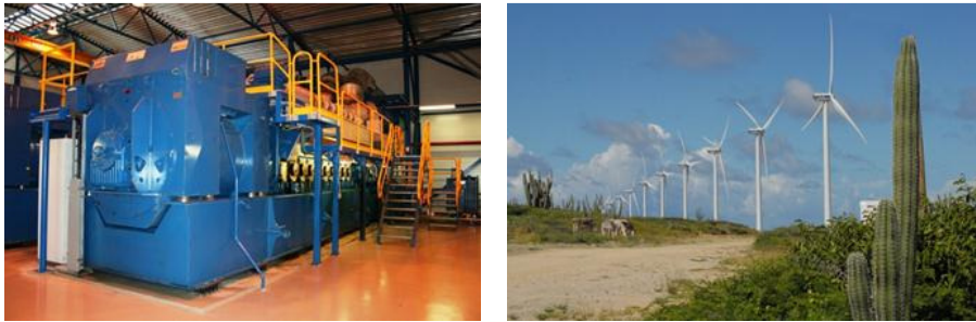
Figure 10.3: The reciprocating engines and the Wind Park.
