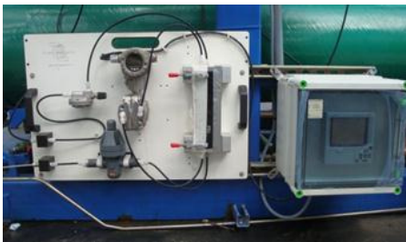
Early Warning System
