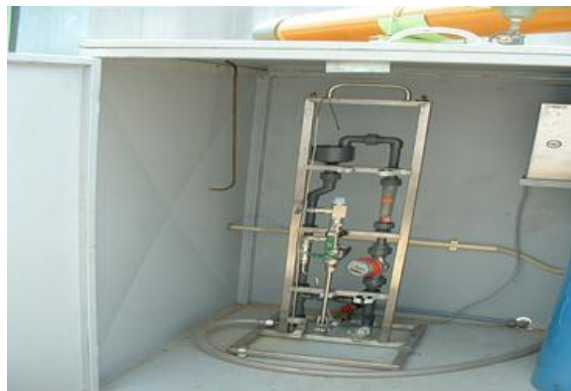
Figure 7.38: The biofilm monitor on the premises of the Desalination Department
