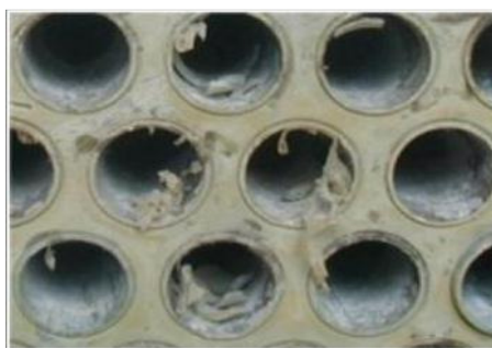
Figure 5.35: Brine heater when on acid dosed operation
