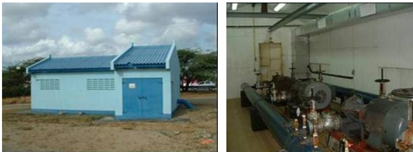
Figure 7.27: The Paradera pump house and distribution pumps
