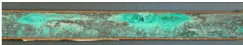
b: practical occurrence of copper corrosion causing blue water
