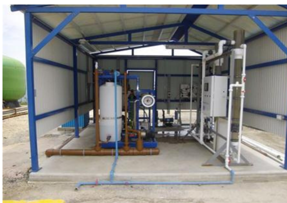
Figure 11.5: A picture of the pilot installation for the drinking water conditioning
